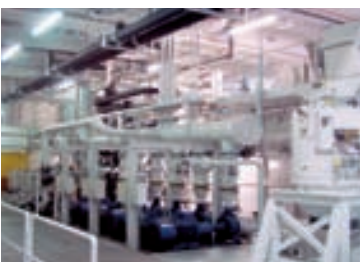
drives as well as for the filtration of coolants in mechanical processing plants.
