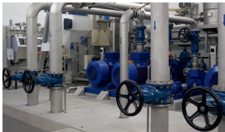
Domestic water supply
